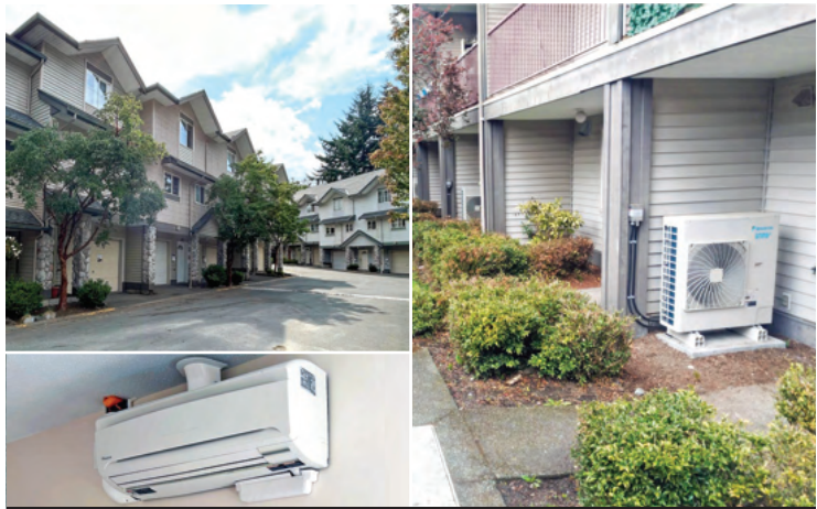
An efficient ductless split heat pump system also provides air conditioning.
